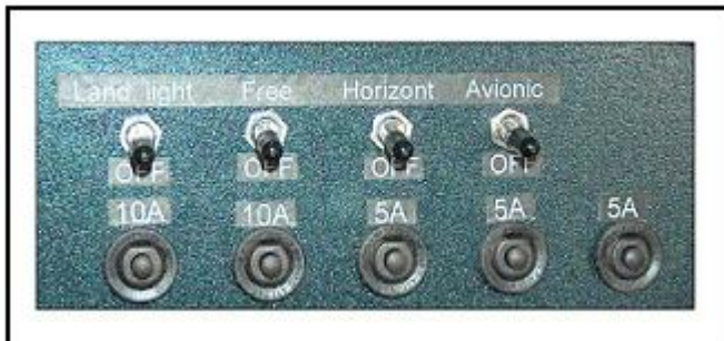
Figure 7 – Switches and fuses panel
